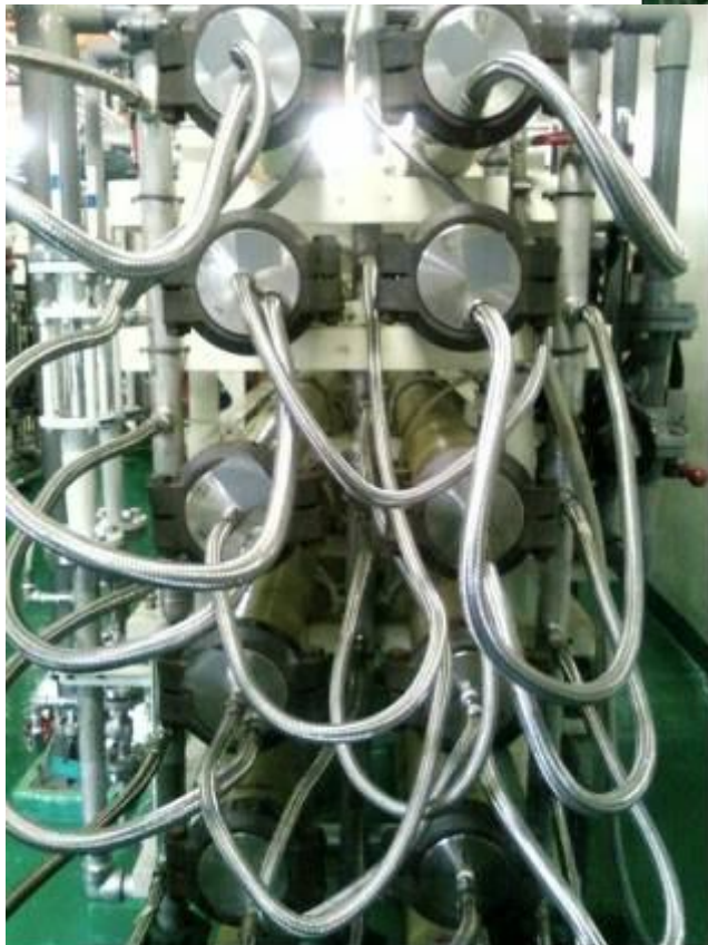
RO SYSTEM CONNECTION
