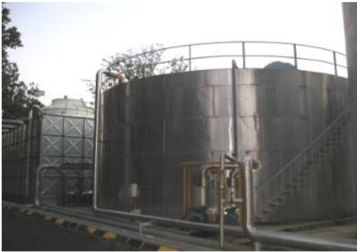
540 M 3 HOT WATER TANK AND 750 M 3 PRESSED WATER TANK
