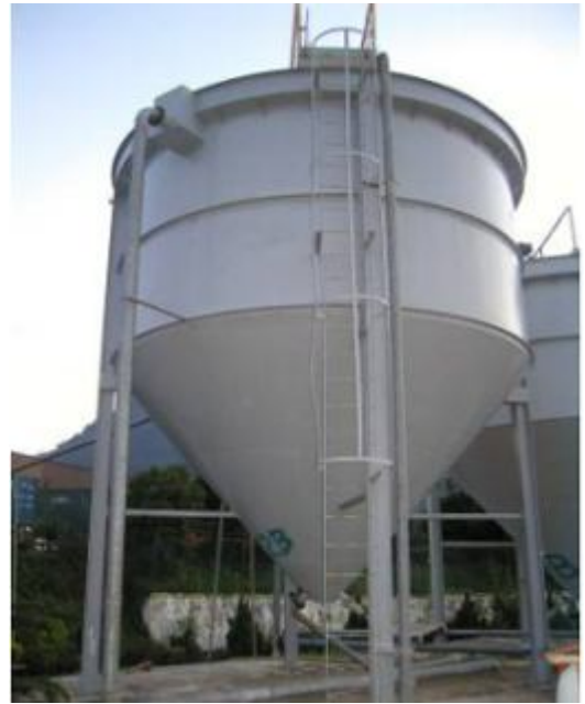
150M 3 MILD STEEL CLARIFIER TANK
