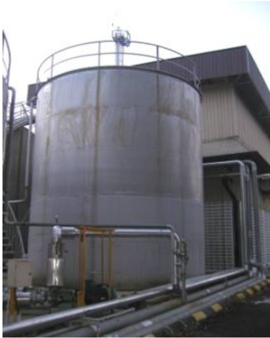
270M 3 SS316L ACETIC ACID STORAGE TANK
