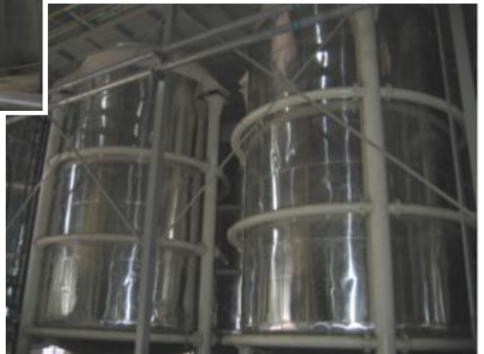
65M 3 MILD STEEL ACTIVATION & COOLING TANKS
