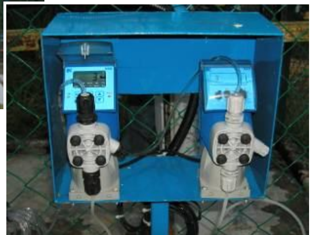
Chemical Dosing Pump
