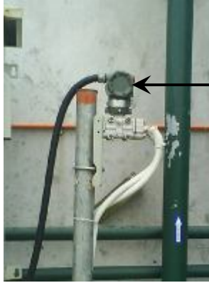
Differential Pressure Transmitter
