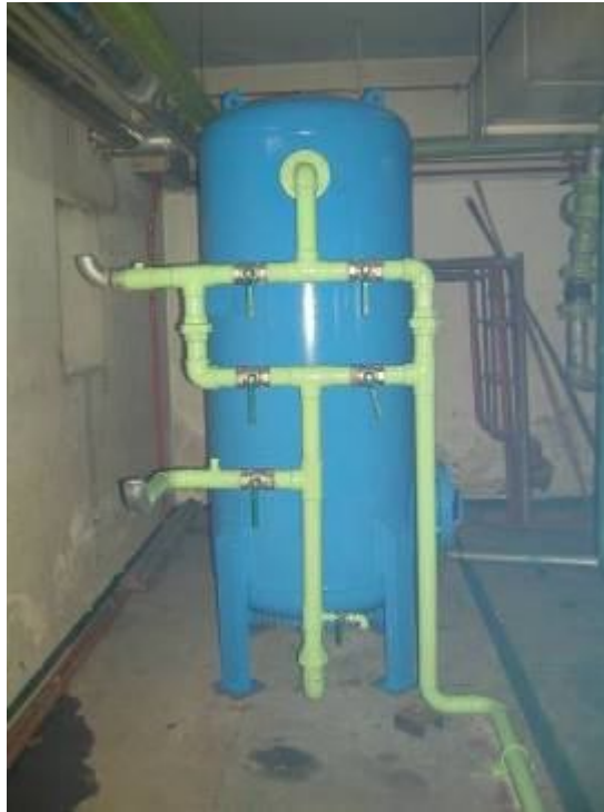
7.5M 3 /Hr - For Filtering Kitchen JBA Water Supply Line
