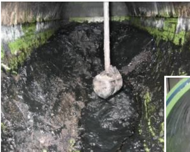
Sludge accumulated inside boiling chamber
